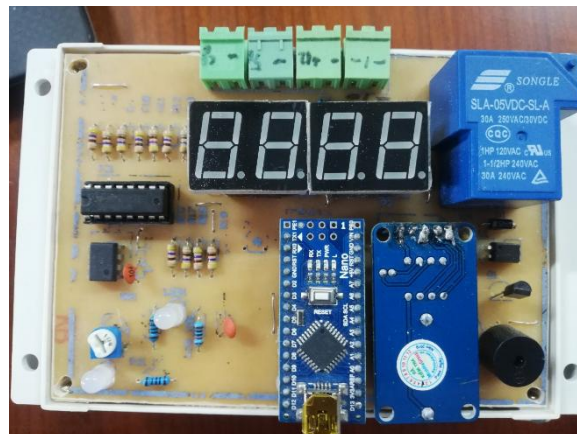
Figure 3. a circuit of the generator battery operation supervision in a BTS station after completion.
