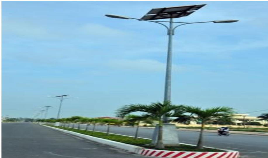
Figure 8. Solar application for street lights
