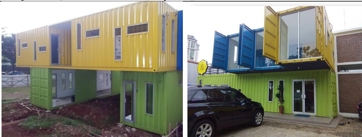
Figure 9 - 10. Assembly and finishing of the building in the field (Courtesy: PT. Magnus Cipta Estetika) (Courtesy: Magnus Cipta Estetika, Pte.Co)
