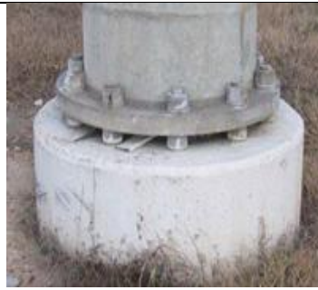
Fig . 1 Base plate bolted to foundation
