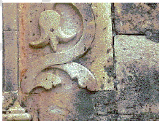
Figure 2 Building damages caused by acid rain, Copala, Mexico [11].
